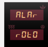
Alarm Burnig pot rotation failure
