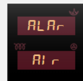
Alarm Air Flow
